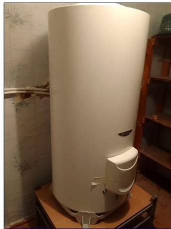
LARGE CAPACITY HOT WATER HEATER TO PROVIDE FOR THE NEW SHOWERS WE INSTALLED FOR THE ORPHANS
