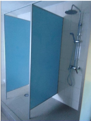
SHOWERS AND HOT WATER FOR THE ORPHANS FOR 1ST TIME
