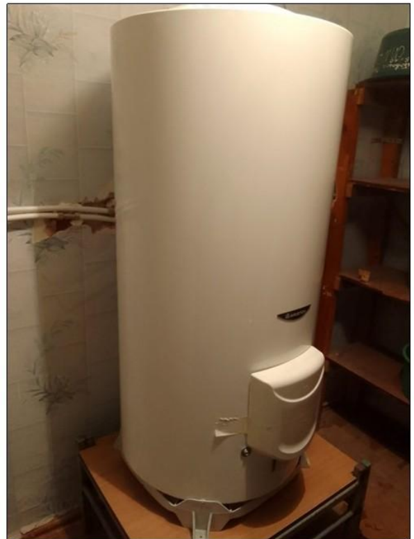
LARGE CAPACITY HOT WATER HEATER TO PROVIDE FOR THE NEW SHOWERS WE INSTALLED FOR THE ORPHANS
